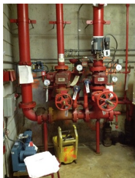
Photo 10: Fire Service and Alarm Valves
