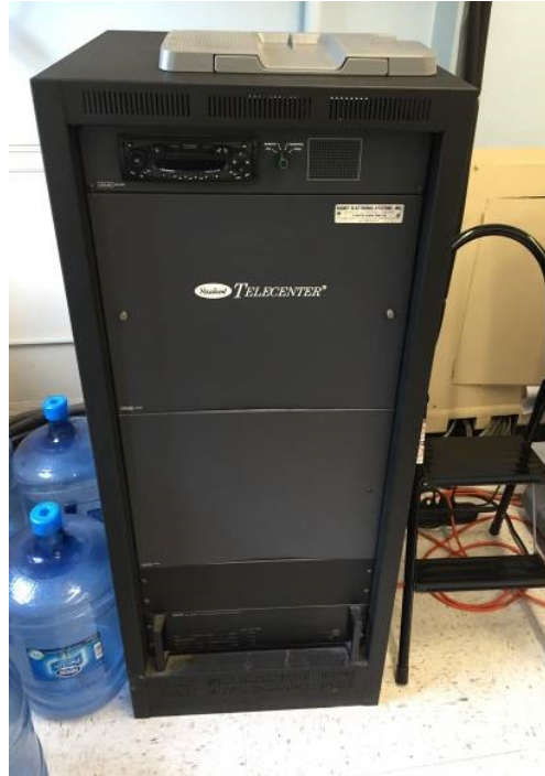
Paging System Headend
