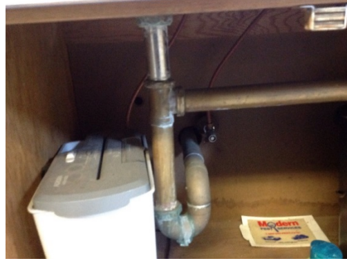
Photo 8: Piping at Classroom Sinks
