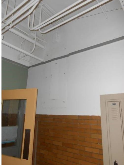
Corridor Mounted Panel
