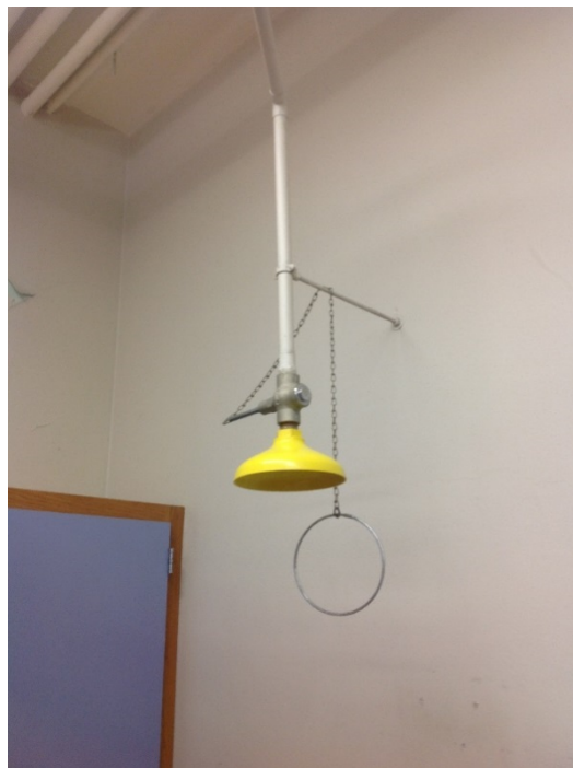
Photo 13: Non-ADA compliant Emergency Shower/Eyewash at Science Labs
