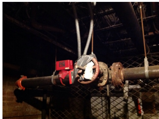
Photo 8: Tamper Switch and Valve in poor condition
