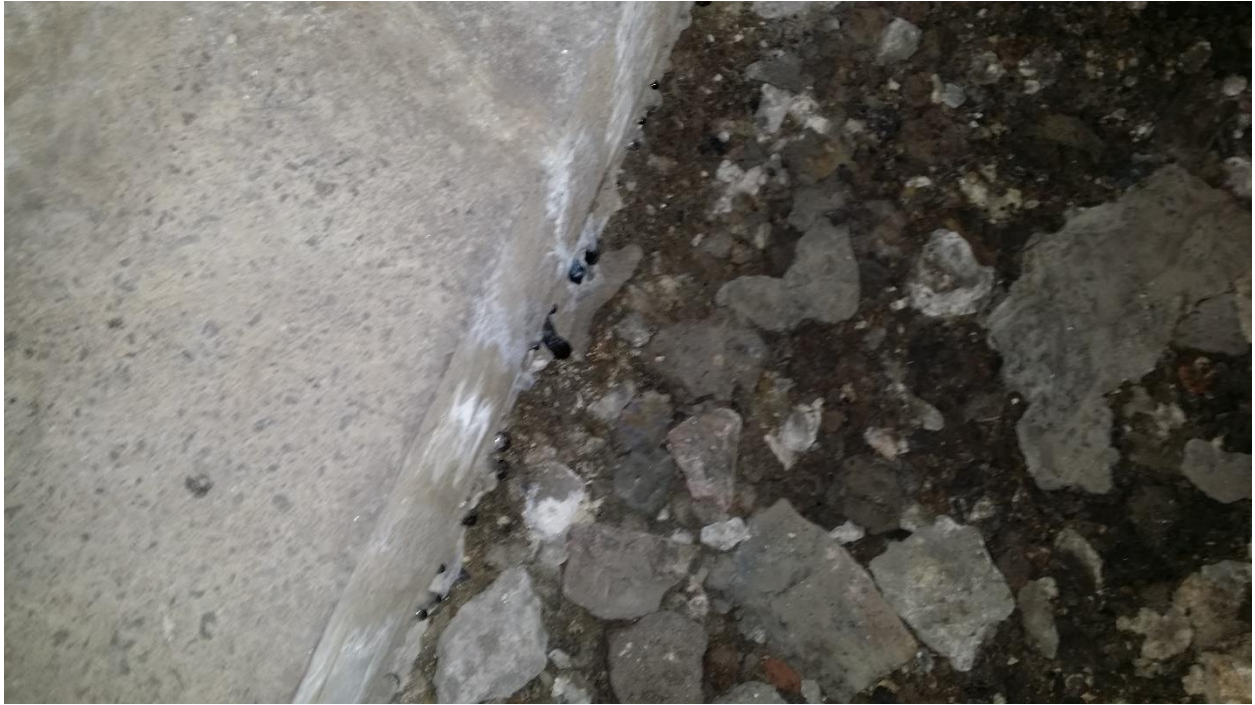
Room off of Boiler Room with Excavation Close up of Ash and Clinkers
