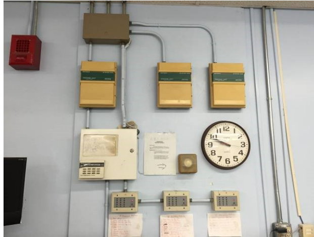
Intrusion Control Panel/Keypad
