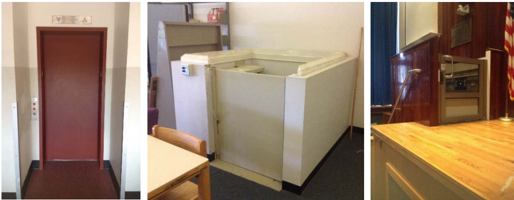
Elevators and Lifts
