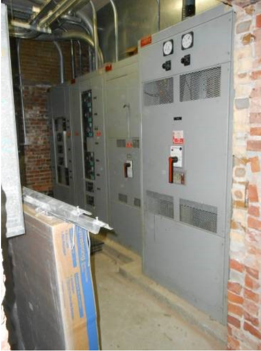
Main Switchboard for Wing D &amp; E
