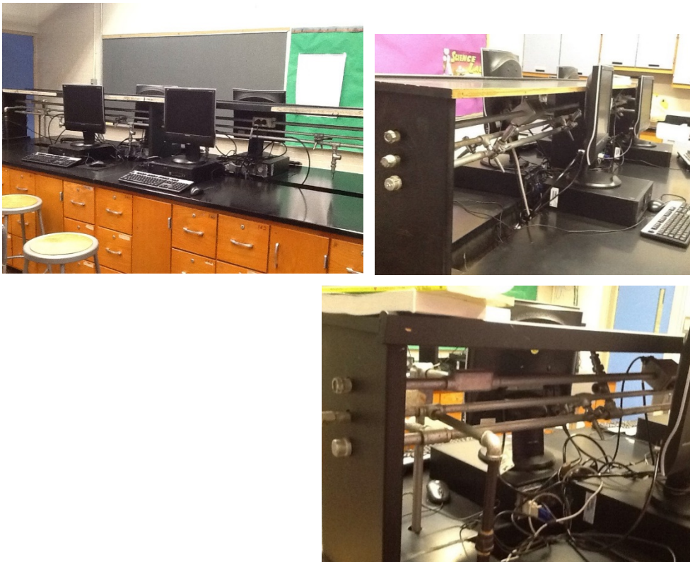
Photo 15: Gas and water piping abandoned in place in Computer Rooms
