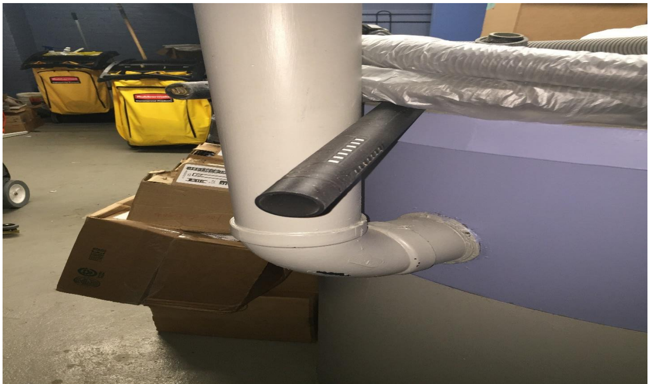
Acid Neutralization Tank in Basement Near Custodial Office
