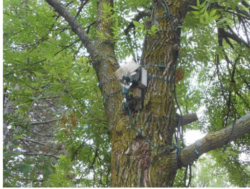
Decorative Tree Lighting Receptacle
