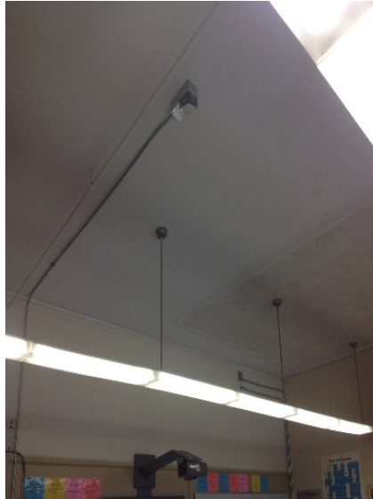
Ceiling Hard Classroom
