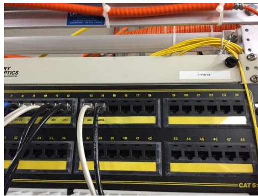
City Hall Fiber Distribution
