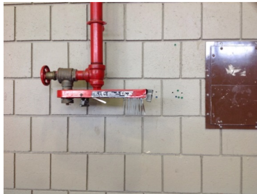
Photo 9: Fire Department Valve
