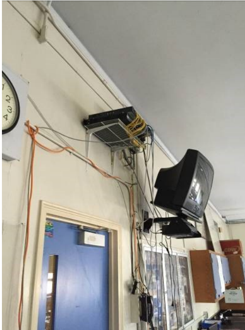
Lack of Receptacles Where Needed
