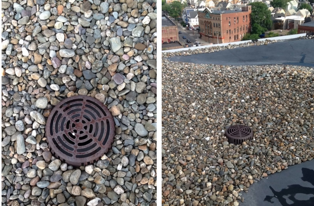
Photo 18: Roof Drains and Domes in poor condition
