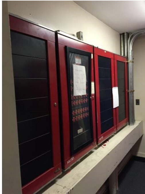
Old Fire Alarm Control Panel
