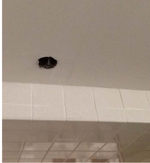
Photo 6: Sprinklers without escutcheon plates
