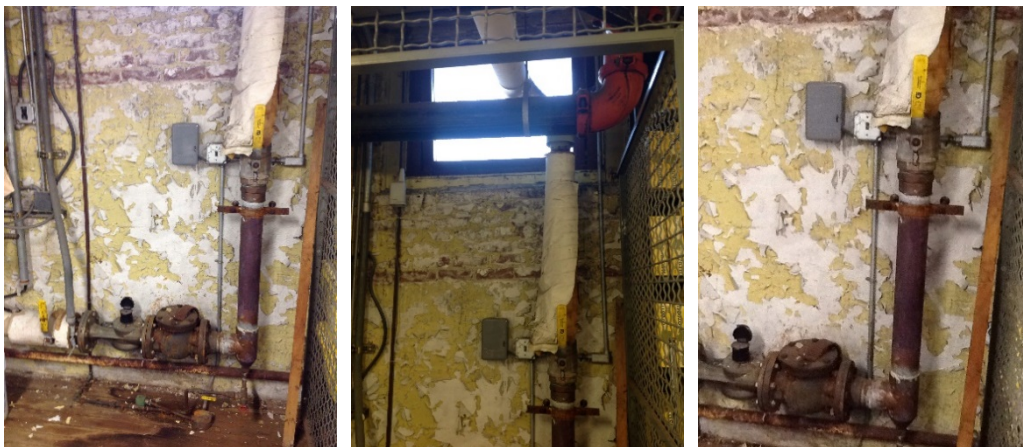
Photo 1: Existing Domestic Water Service
