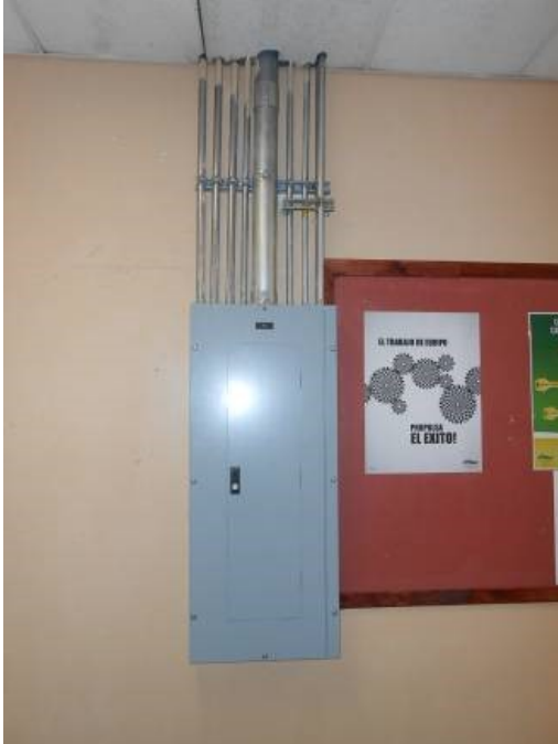
Upgraded Surface Mounted Panel
