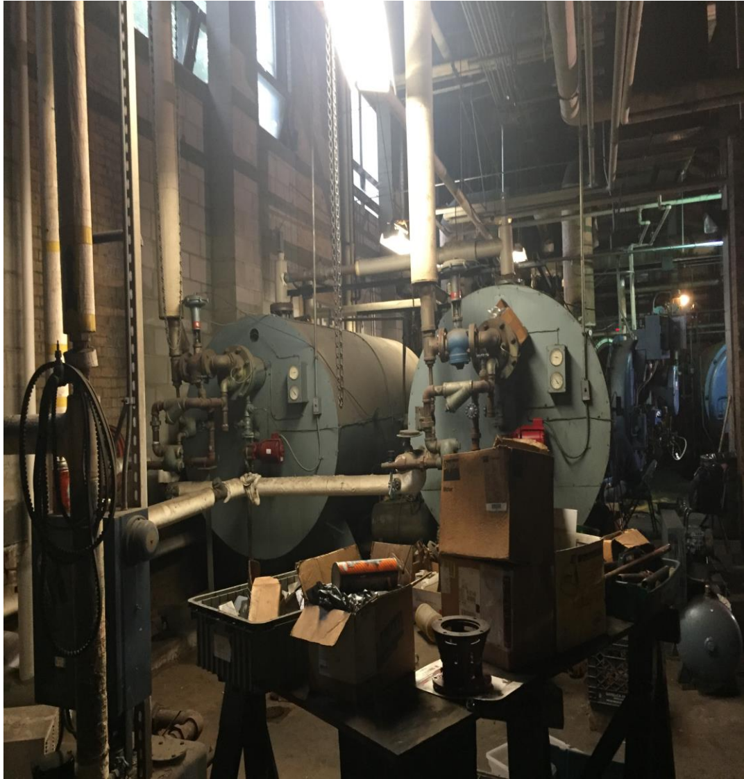
Boiler Room with Fiberglass Pipe Insulation
