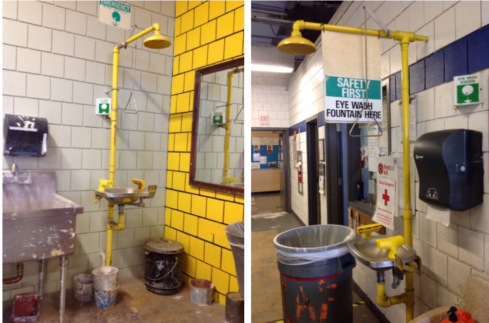
Photo 14: Non-ADA compliant Emergency Shower/Eyewash at Auto Shop
