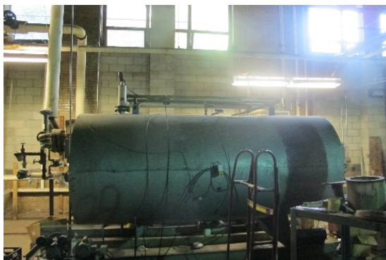
Photo 3: Steam-Fired Storage tanks
