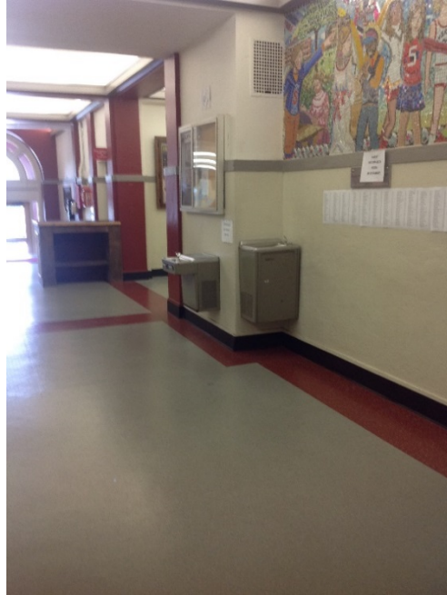
Photo 22: Existing drinking fountains
