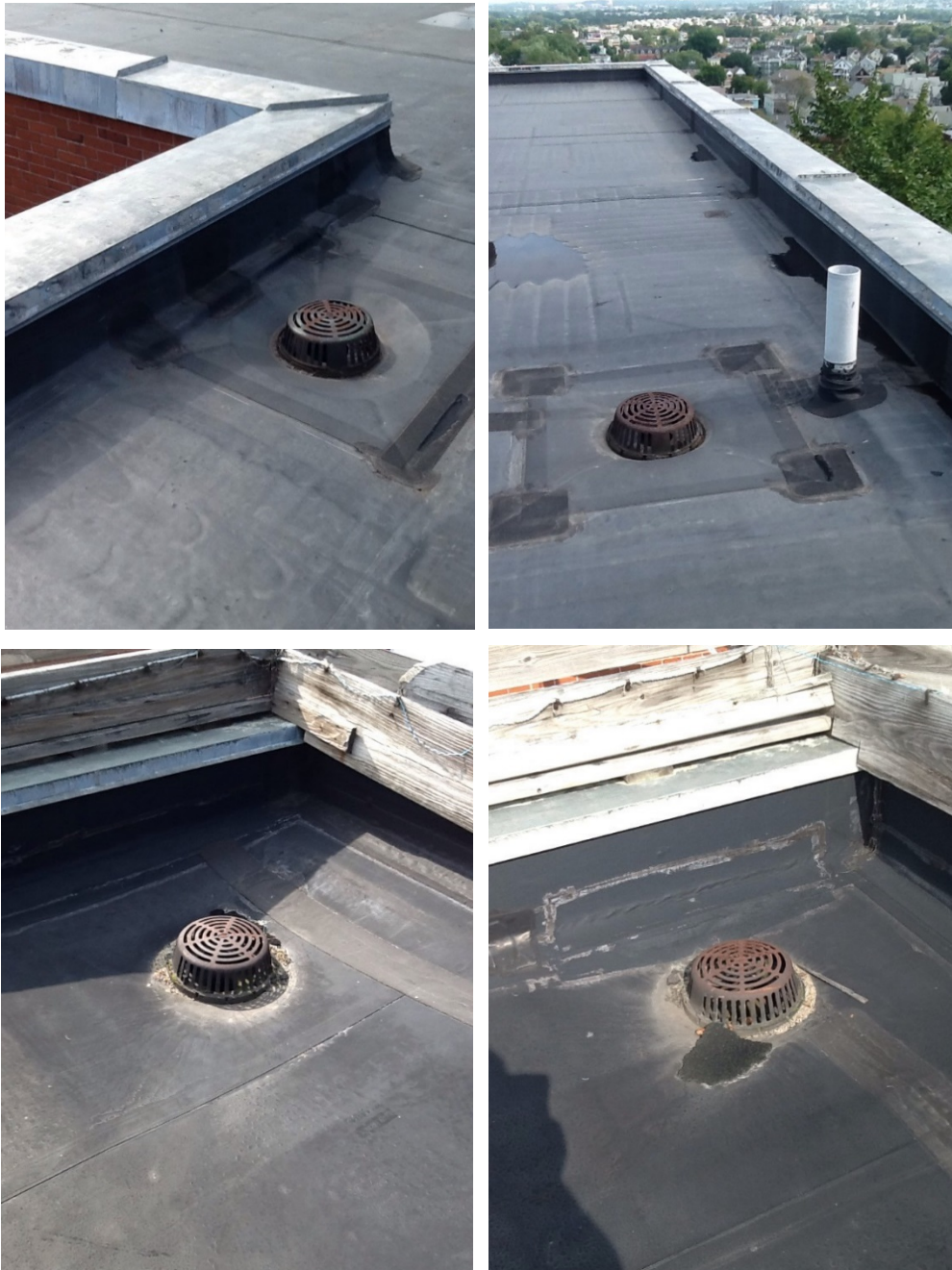
Photo 17: No Overflow Drains installed.
