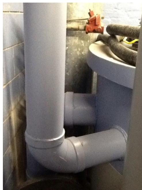
Photo 11: Existing Limestone Chip Tank
