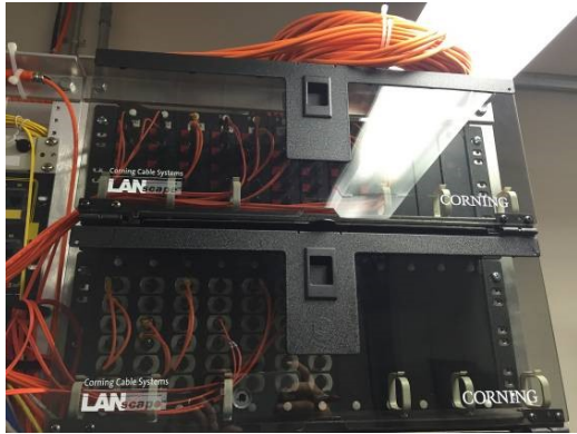
Building Fiber Distribution
