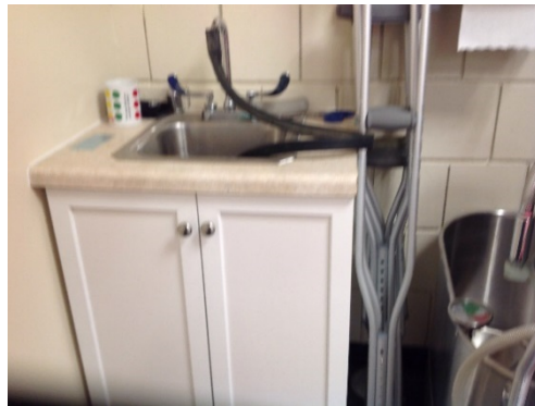
Photo 23: Non-ADA compliant sinks
