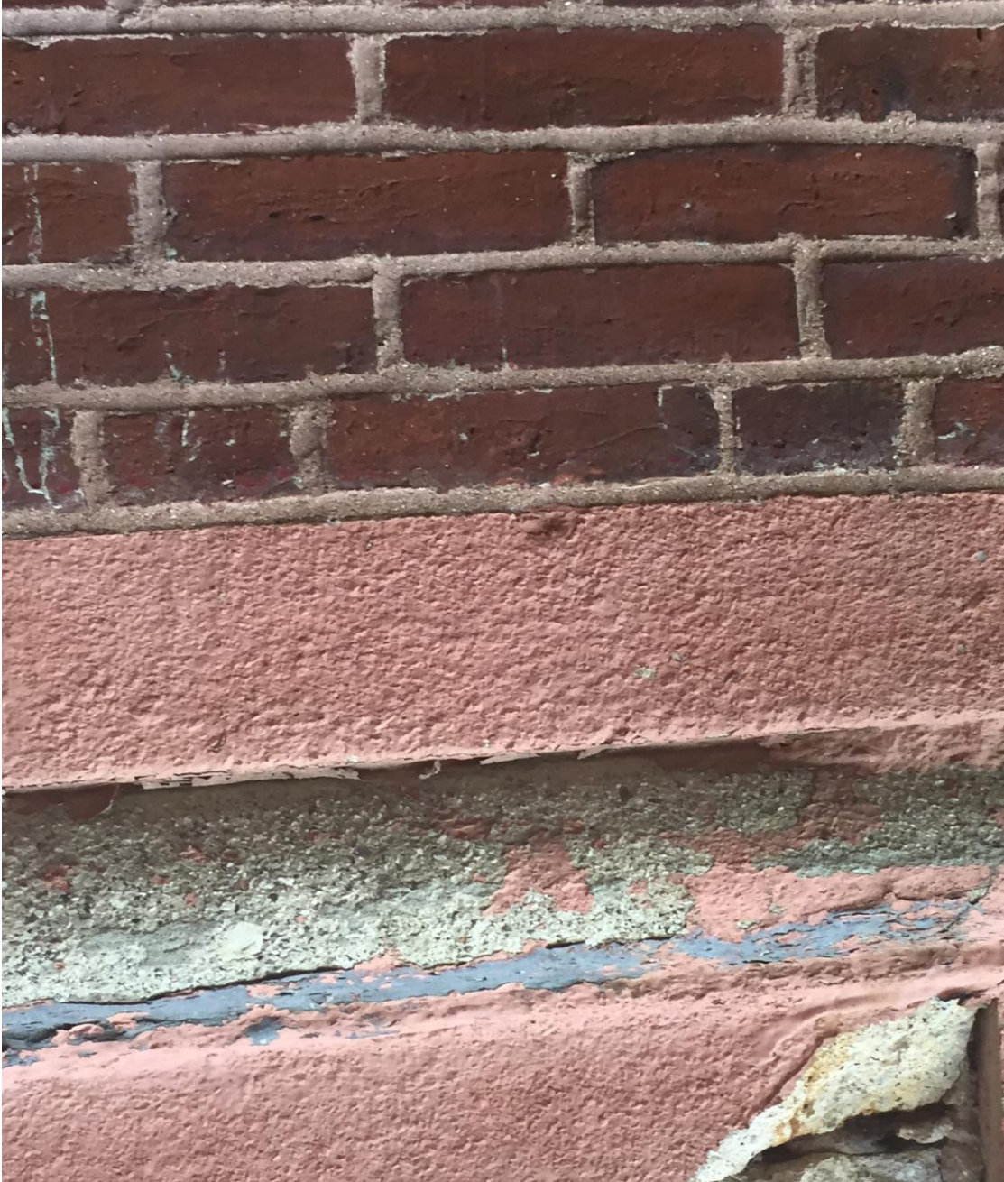
ACM Tar on Coping 1929 D Wing
