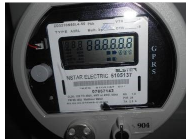
Wing A, B, C Meter
