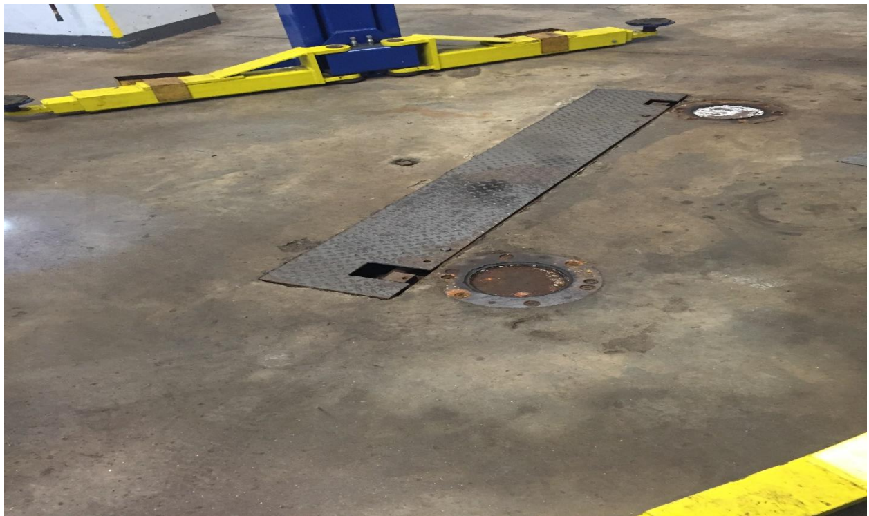
Old Hydraulic Lift with Reservoir Auto Shop
