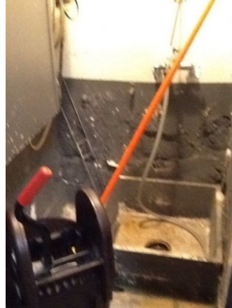
Photo 2: No backflow preventer for detergent at mop receptor
