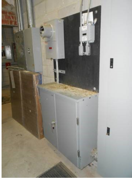
Meter and C.T. for Wing D &amp; E
