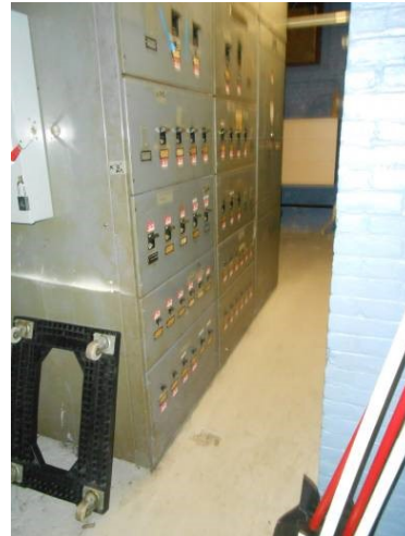
Main Switchboard for Wing A, B, C
