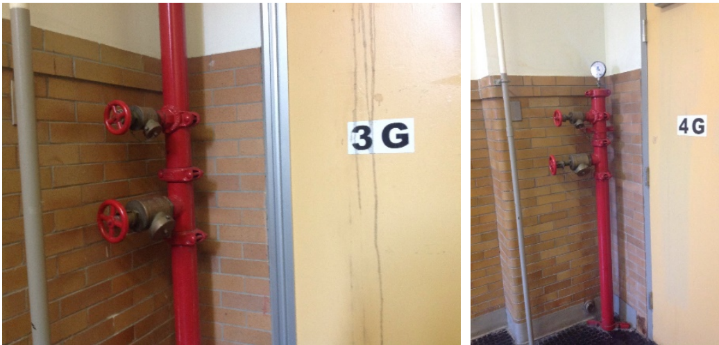
Photo 1: Existing Standpipes with FDV's at Stairwells (Typical for A, B & C Wings)
