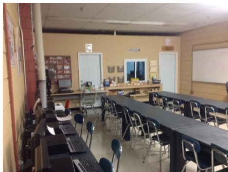
Photo 11: Sprinklers not code compliant
