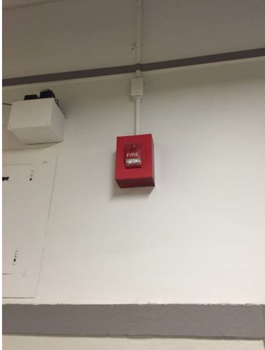
Typical Notification Appliance
