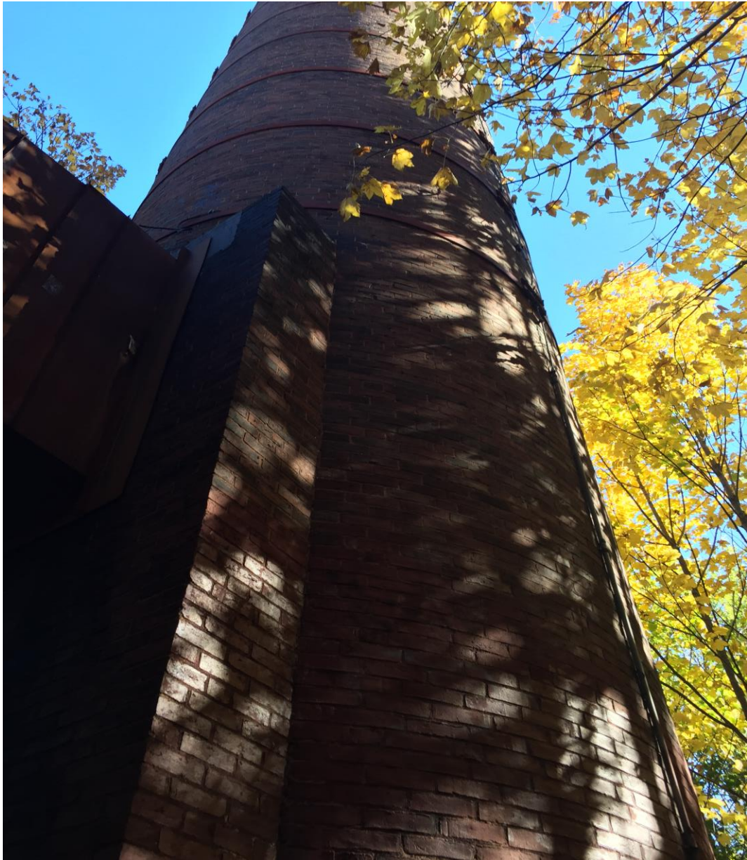
Older Chimney With Possible ACM
