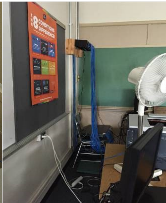
Typical Computer Switch
