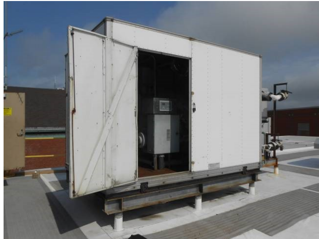
Roof Mounted Generator
