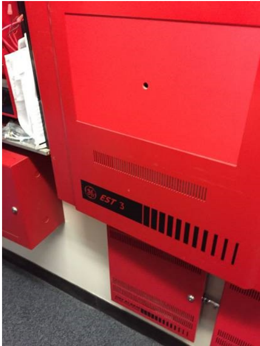
Fire Alarm Control Panel
