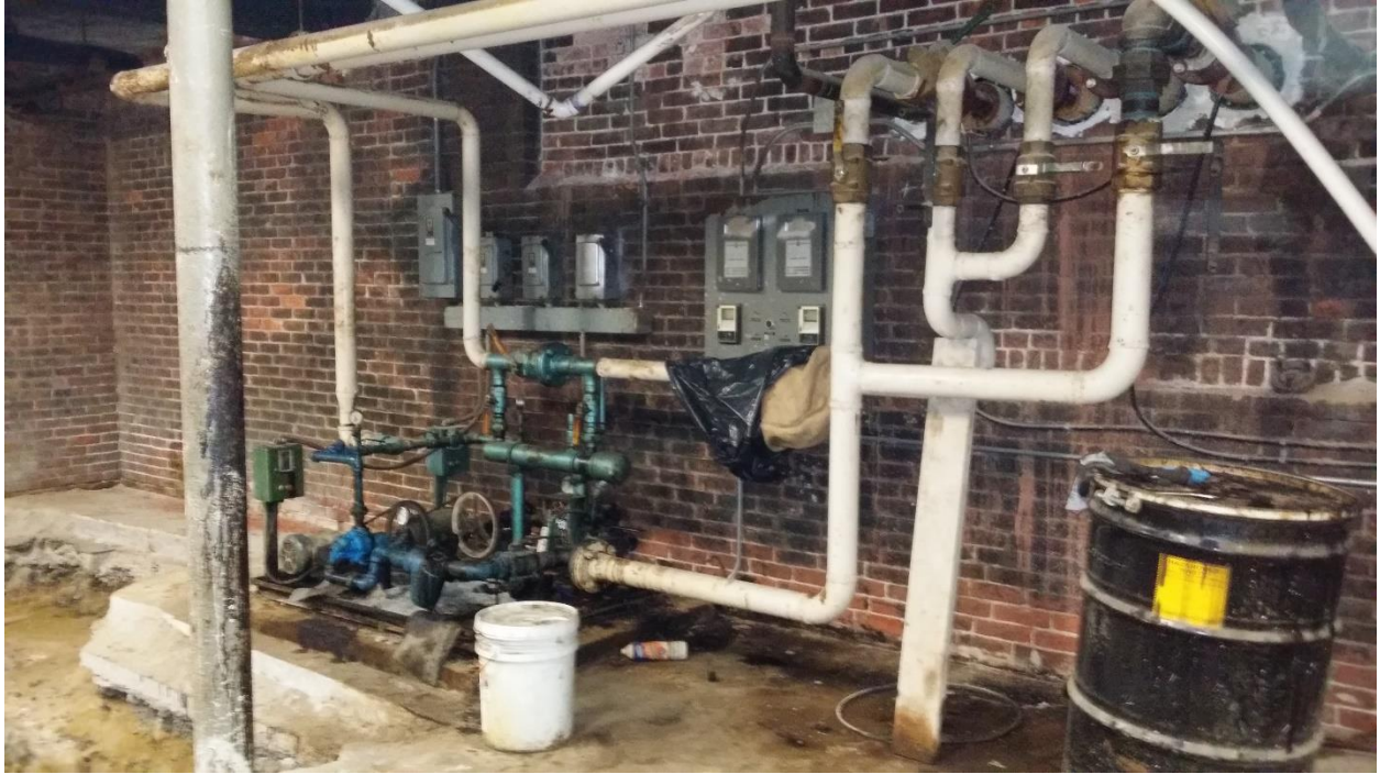
Drum with Hazardous Waste Sticker off Boiler Room
